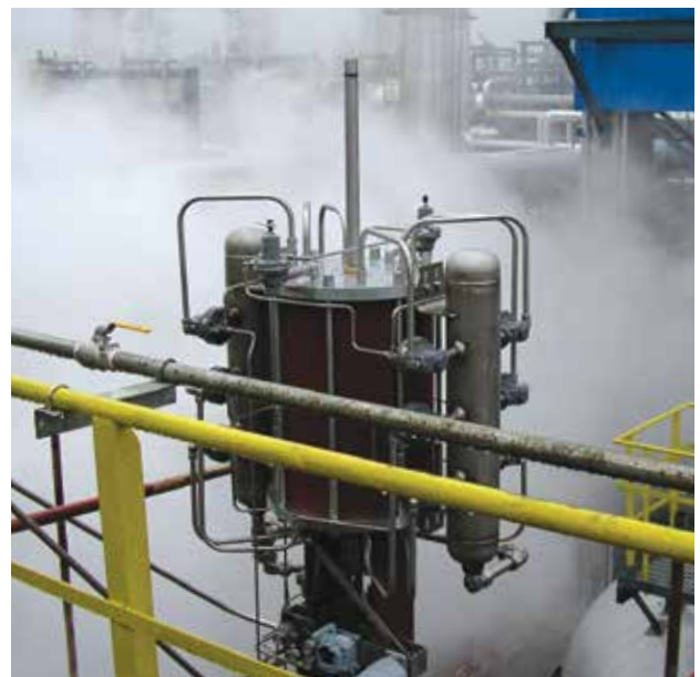
SVI II AP on steam conditioning valve
