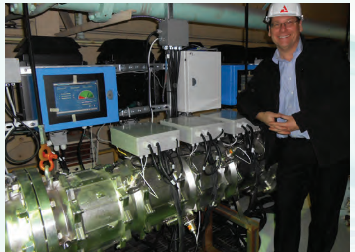
Atlantium Hydro-Optic Dechlorination installation at Plant Bowen, Georgia USA
