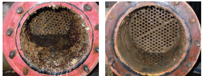
Mussel settlement in cooling water pipe before and after water treatment with Atlantium UV
