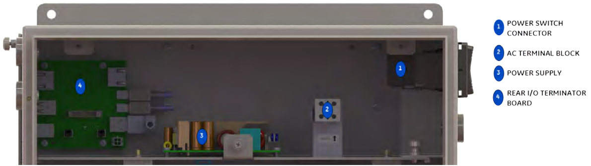
Figure 43: Electronics Enclosure (Top Shelf) — Sievers M5310 C On-Line TOC Analyzer
