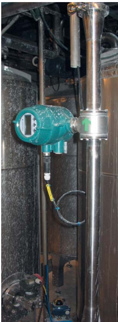
Flowmåler monteres vertikalt for at undgå luft i systemet.
