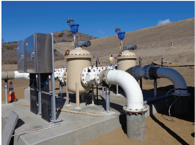
A view of the control panels on a 14" automatic strainer removing zebra mussels from lake water
