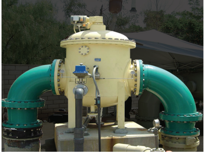
16" automatic strainer removing quagga mussels from lake water
